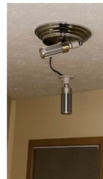
Figure 2: Use of existing fixture of mudroom (or any other closed room) for ultraviolet light disinfection.
